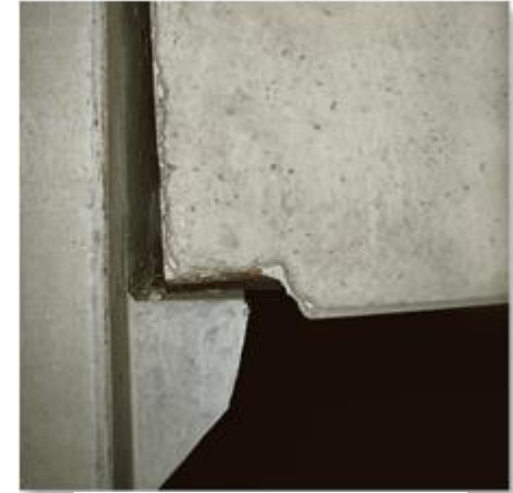
This concrete girder rests on the ledge that is assumed to act as a smooth contacting surface. (5)
